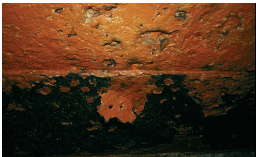
Figure 5 Corrosion at metallic anode sites and spalling of the corrosion product/paint layer.
